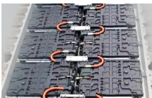
Battery charge/discharge test
